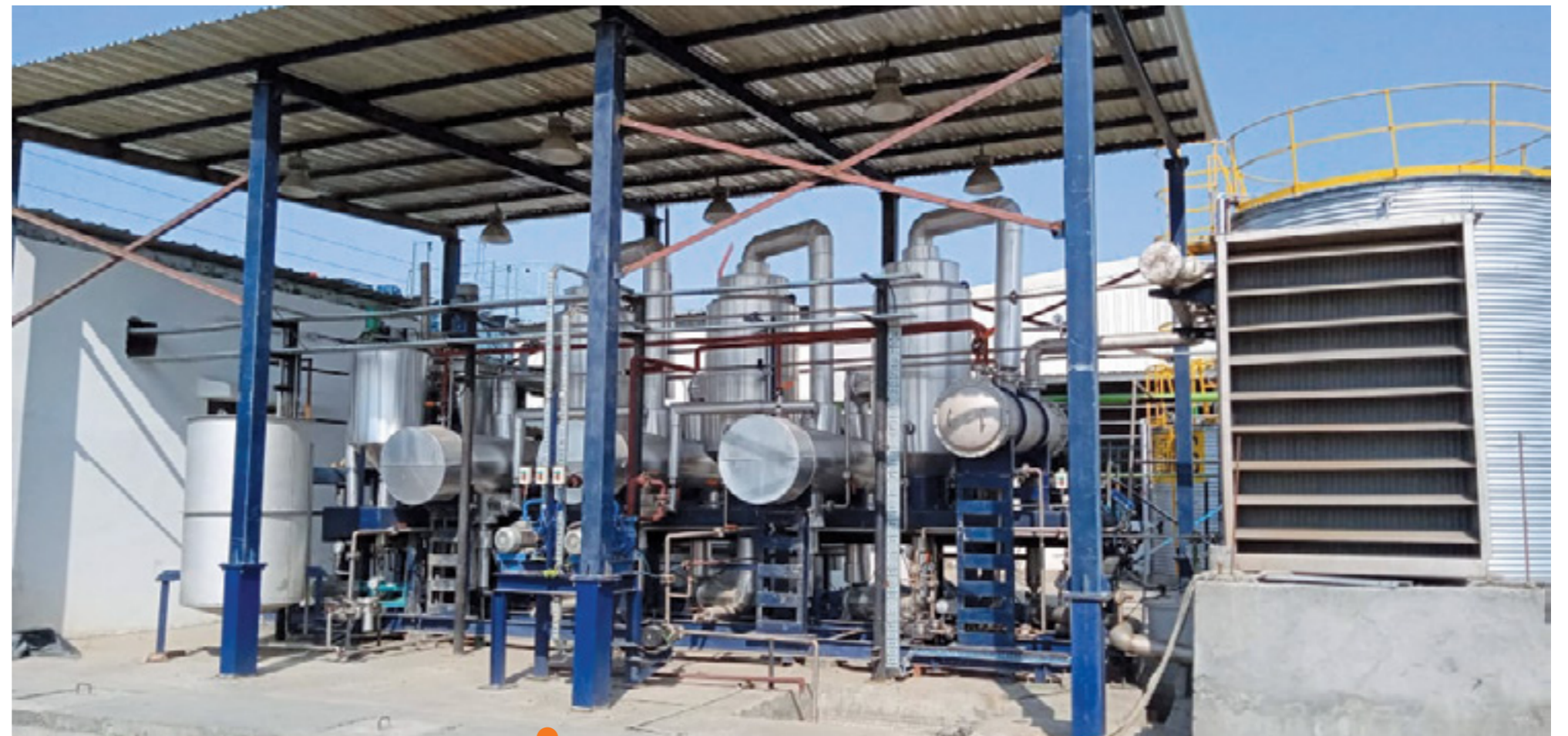
Zero Liquid Discharge (ZLD) Effluent Treatment Plant
